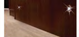
Courtesy LED lighting
